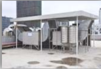
Paint Shop Ventilation
