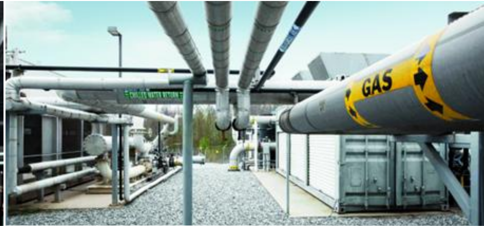
Methane gas at Spartanburg plant
