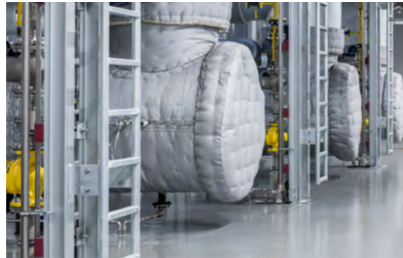
New combined heat and power systems at the BMW plants in Dingolfing and Landshut in Germany: compared to conventional technologies, the CO 2 savings will amount to 75,000 tonnes per year. For this contribution towards environmental protection, the Group plans to invest around €90 million in total at the two locations.
