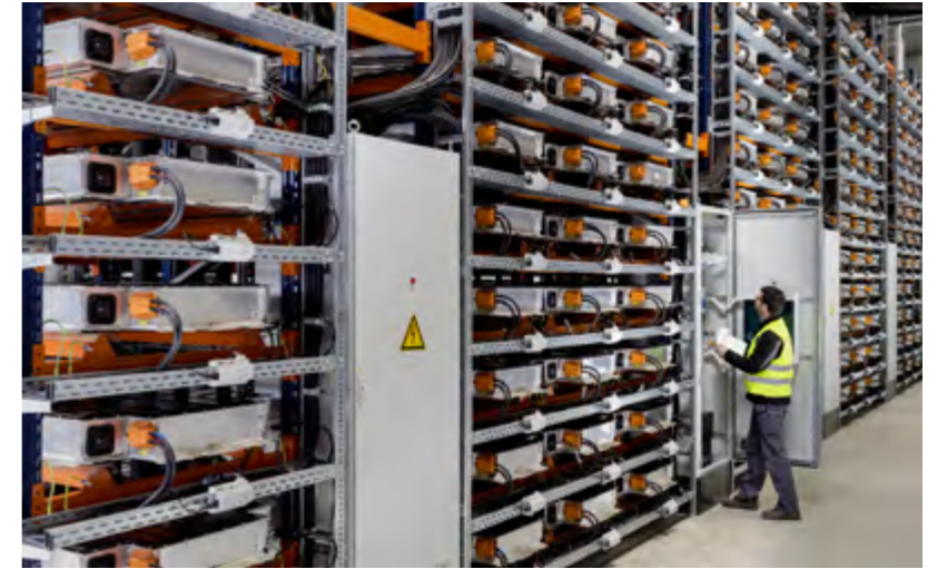
Innovative, sustainable and profitable second-life use of car batteries: the BMW Group's storage farm in Leipzig.
